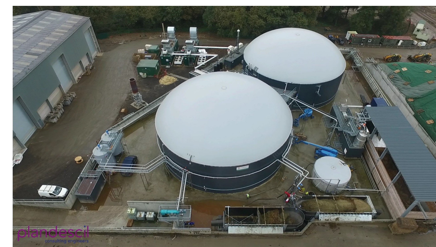
Example AD plant
